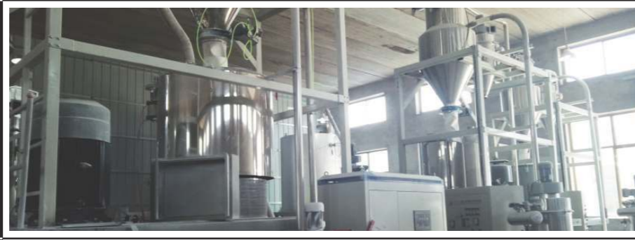
1 Raw material mixing system
